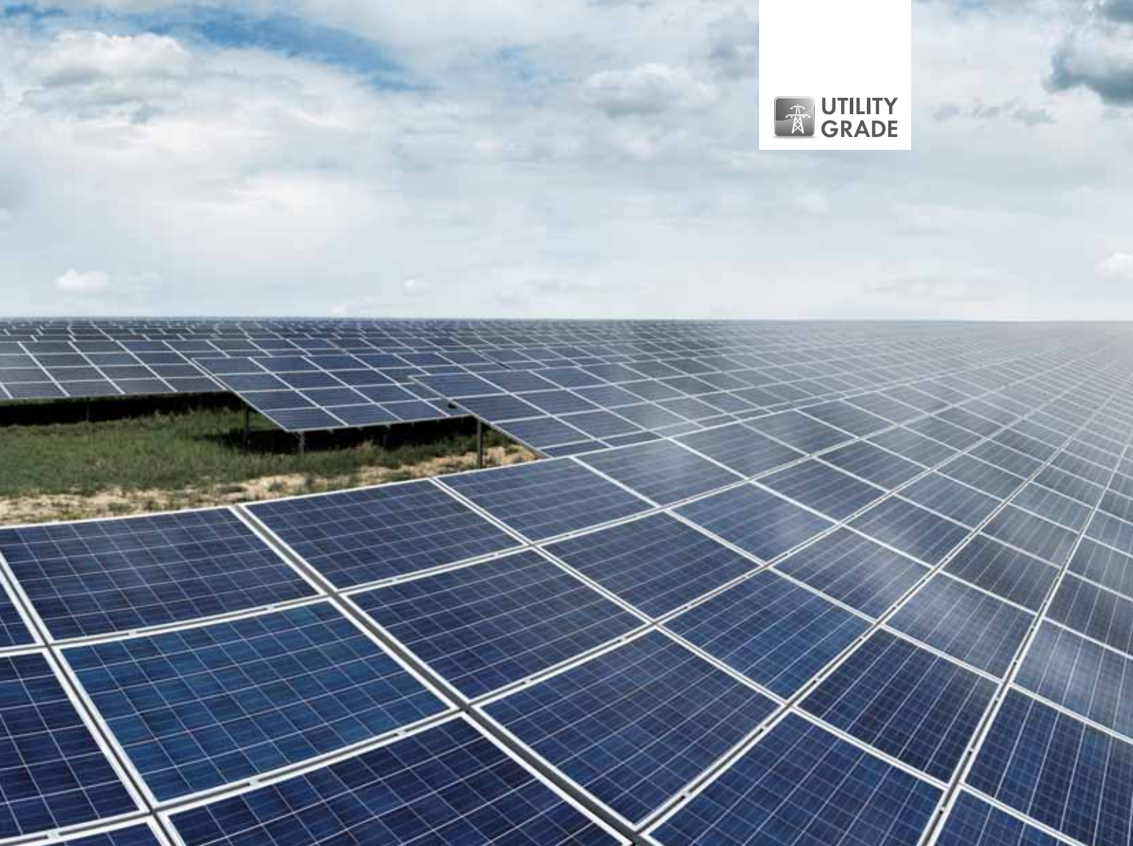
Heideblick PV farm, Gahro Military Airfield, 27.5 MW, project implemented by Enerparc (Sunny Central CP inverter)
